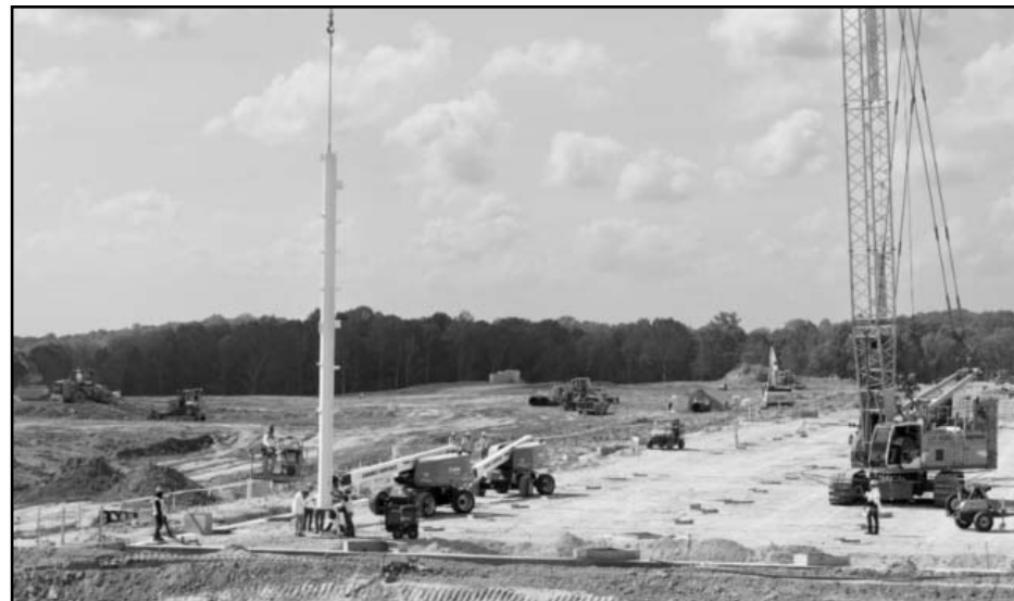
The BMW Group held a ceremonial beam signing celebrating the first beam erected onsite at Plant Woodruff on October 5th. BMW photo
