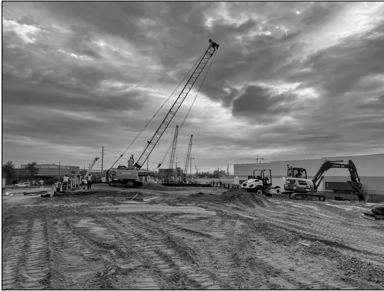
Construction progresses at the Navy Base Intermodal Facility in North Charleston, South Carolina. (Photo/SC Ports/Walter Lagarenne)
