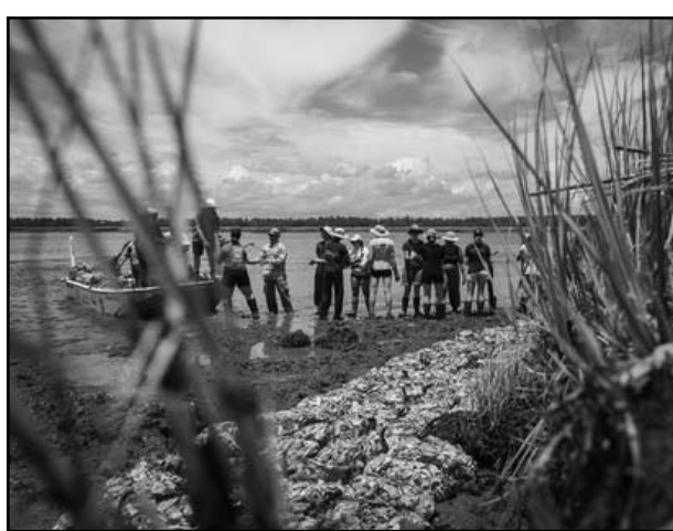
Volunteers form an assembly line to move bags of oyster shells into place along the shoreline. (Photo: Kaitlyn Hackathorn/SCDNR)
